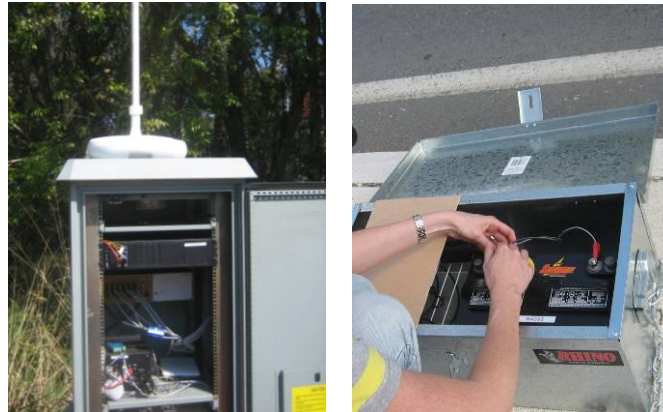
Figure 2: Typical MAC reader deployments in cabinet (left) and with battery (right)
