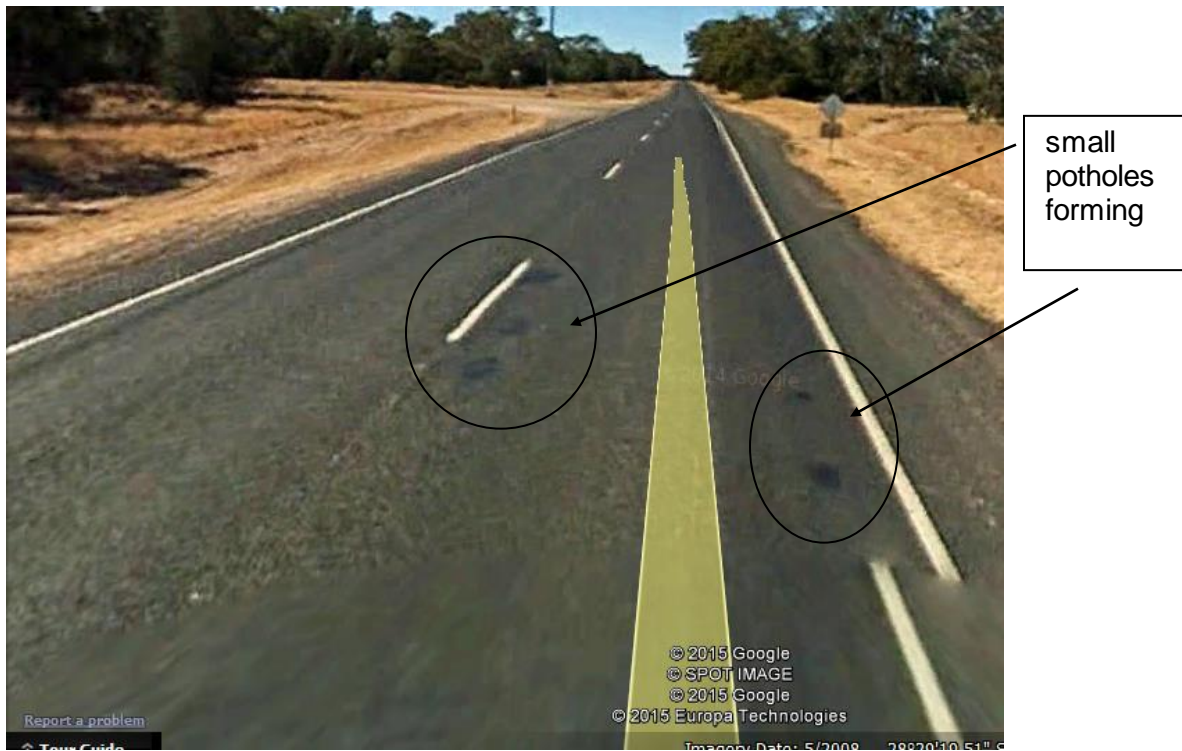
Figure 9: The Cunningham Highway looking east (ref: Figure 6) showing small potholes forming (courtesy: Google Earth)
