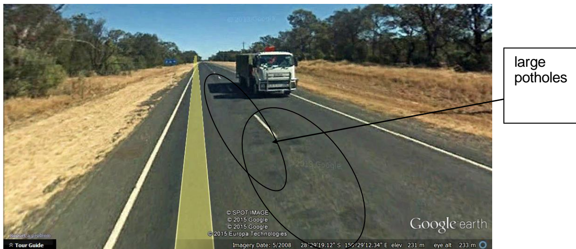
Figure 10: The Cunningham Highway looking west (ref: Figure 7) showing series of larger potholes (courtesy: Google Earth)
